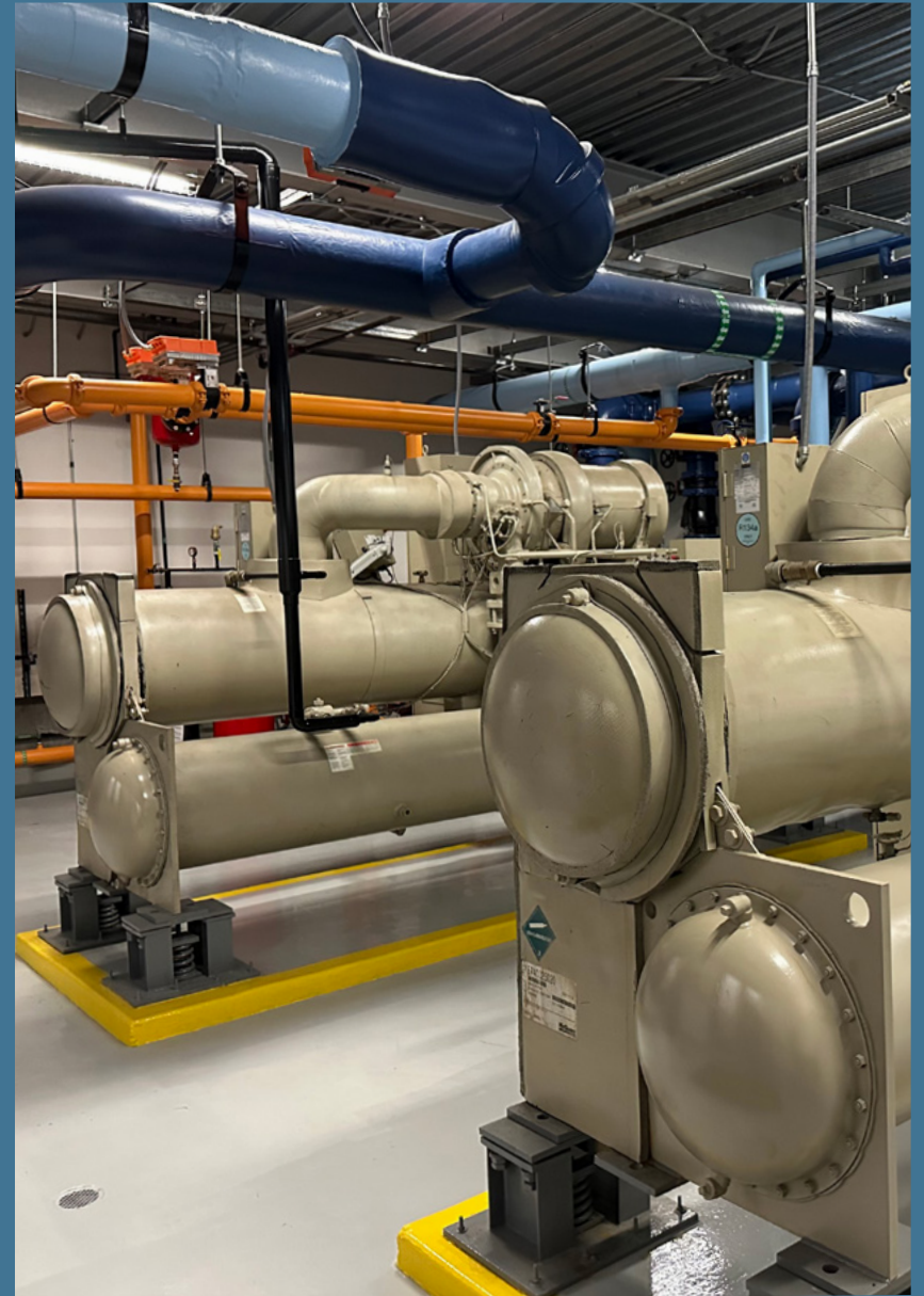
12400 High Bluff Drive, San Diego Mechanical Room
